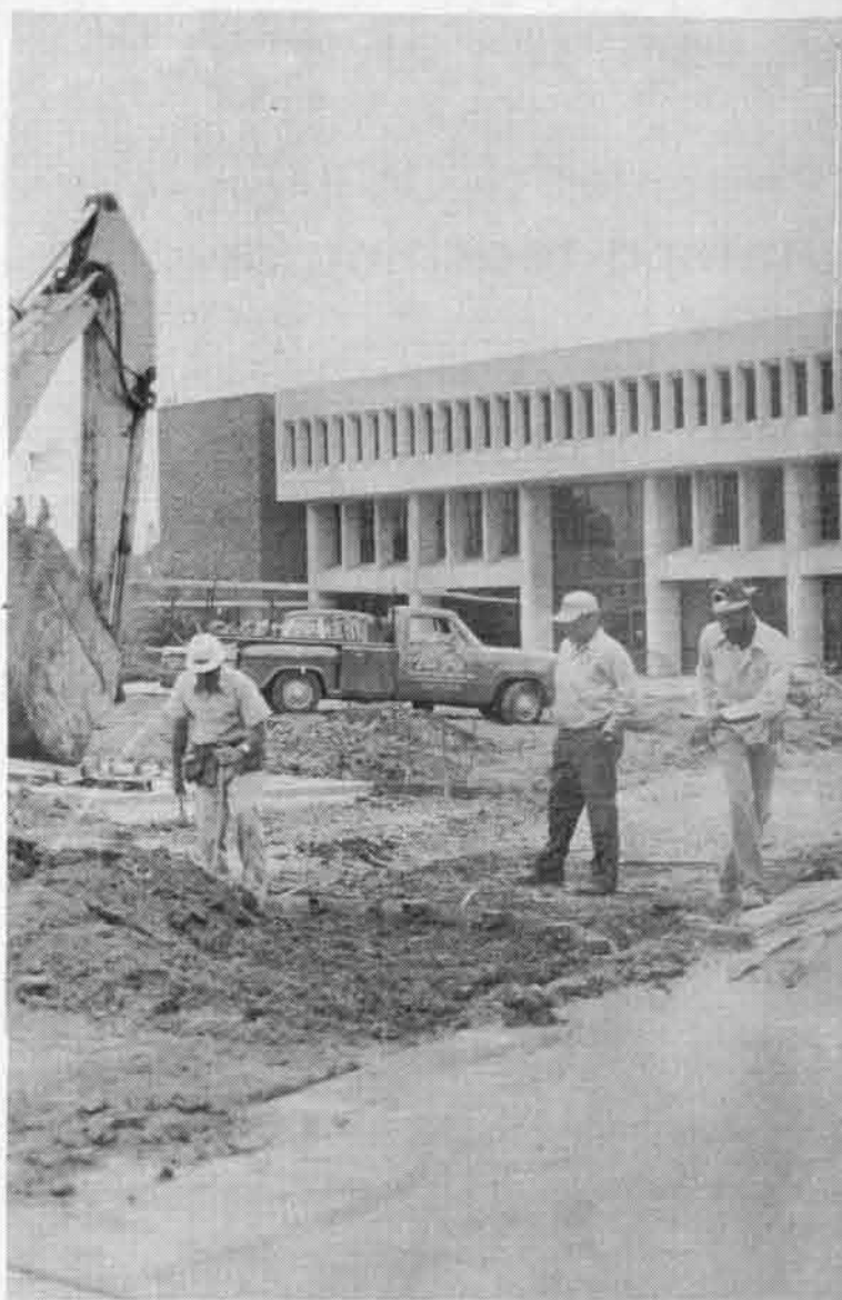
COMMONS KNOWLEDGE: Workmen construct one of the many paths that will connect buildings across the Commons area. The landscaping, which was scheduled for completion last fall, was delayed by poor weather. Work on the project is slated to end in four to six weeks [photo by Earl Swift].
